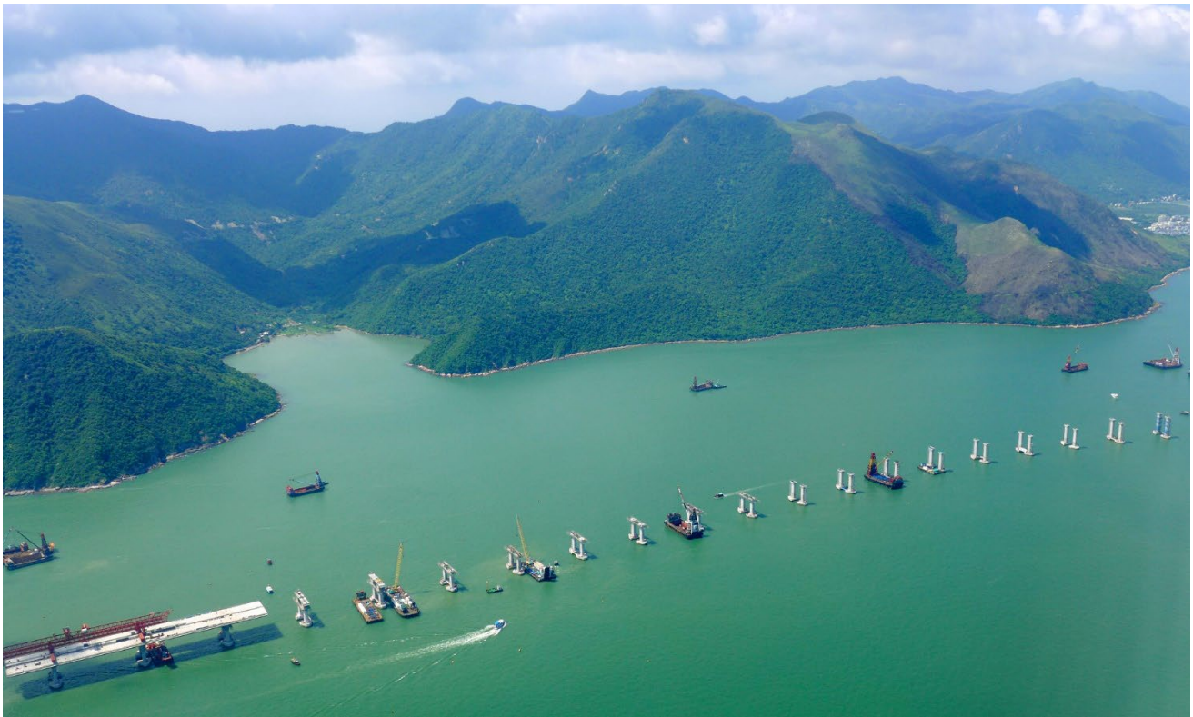
Figure 2. The Hong Kong section of the Hong Kong-Zhuhai-Macau Bridge under construction in 2015 off the coast of Lantau Island. (Image Credit: Wikicommons)
